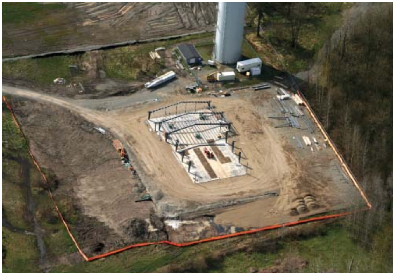
Currently under construction, the new Muckleshoot Water Treatment Facility will come on line later this year.
